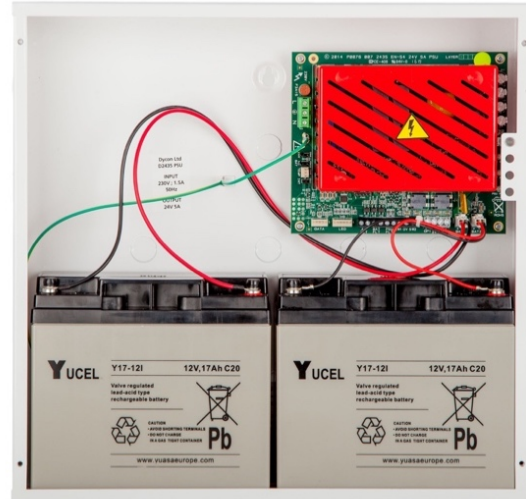
EN54-17 box fitted with D2435-17, 5A PSU & 2 x 17Ah batteries
